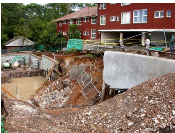
Figure 4.4.2.1: Excavation failure at Beecroft.
