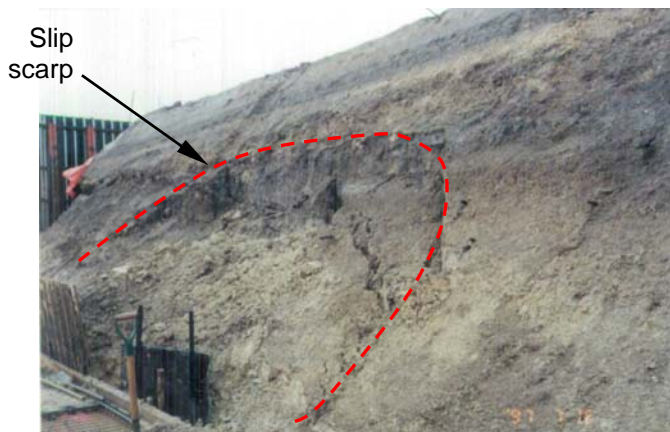
Figure 4.4.1.4: Batter failure during construction.
