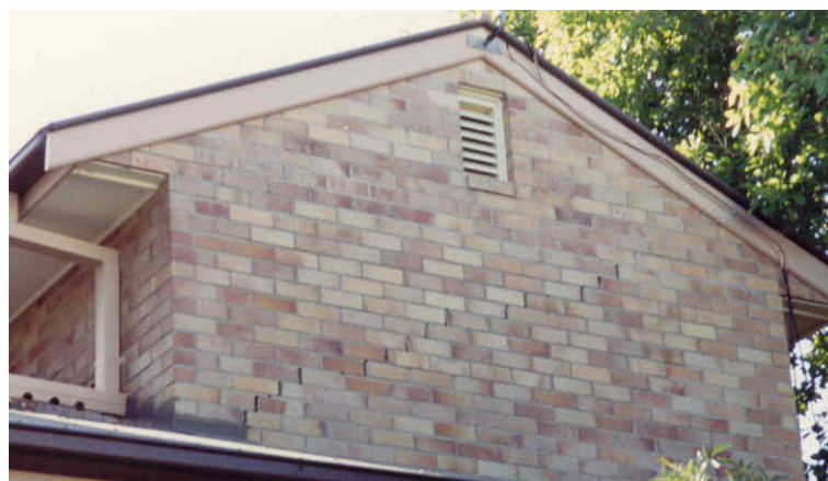
Figure 3.6: Diagonal, step-wise cracking on external brickwork of house.
