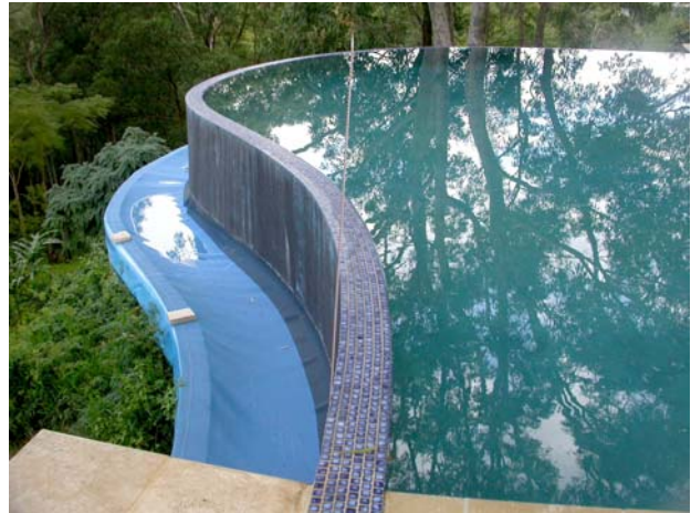
Figure 4.3.2: No 'wet-edge' due to the pool settling.
