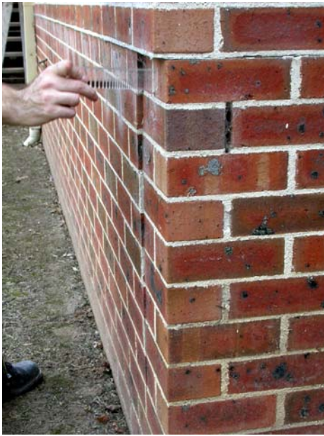
Figure 5.2.2: Horizontal separation of brickwork.
