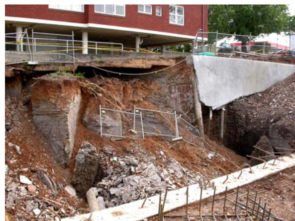
Figure 4.4.2.2: Excavation failure at Beecroft.
