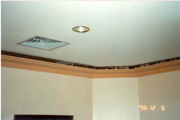
Figure 3.2: Separation of cornice from ceiling.
