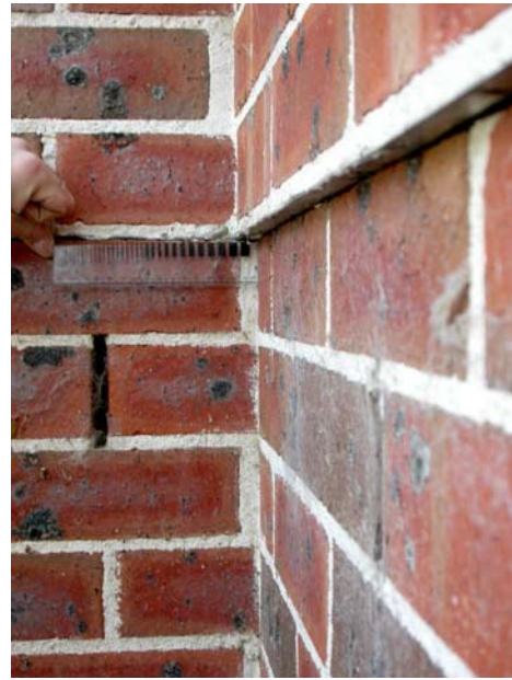
Figure 5.2.3: Horizontal separation of brickwork.
