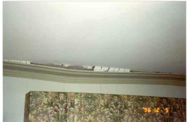
Figure 3.3: Separation of cornice from ceiling.
