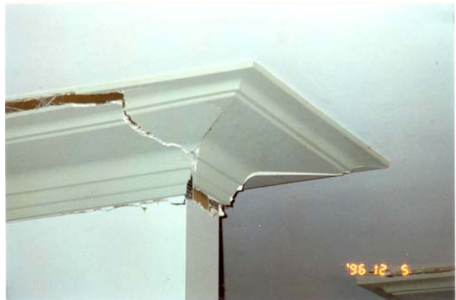
Figure 3.5: Detail of separation of cornice from ceiling.
