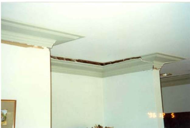
Figure 3.4: Separation of cornice from ceiling.
